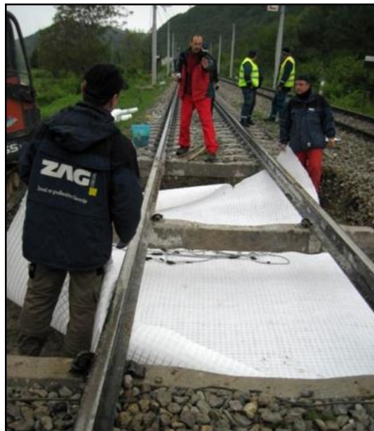
Figure 2: Construction of test site in Sava exit (Slovenia) for SMART RAIL project. Placement of geocomposite at the top of the subgrade.
